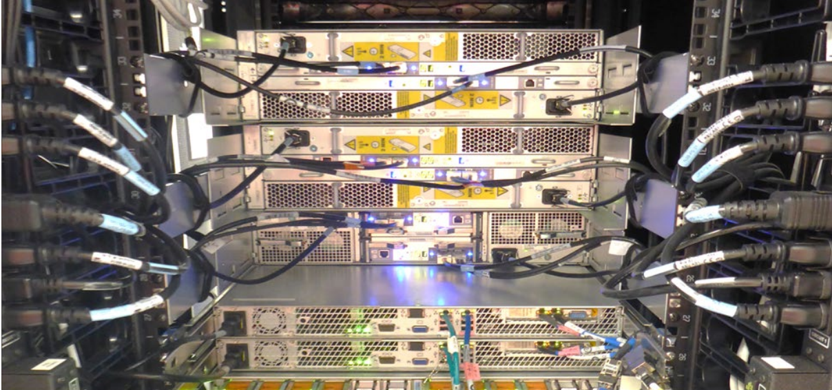
Figure 1: Server Cabinet with Power Distribution Units on Both Sides of Chassis
