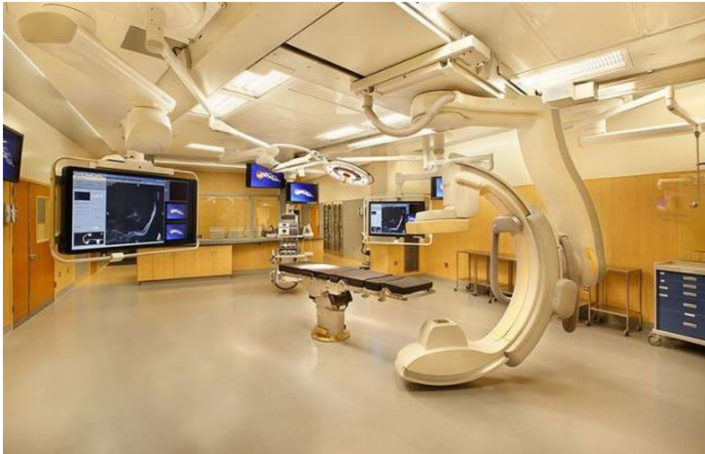
PRIOR TO PROCEDURE OPERATING ROOM, MONOPLANE HYBRID 900 NSF
