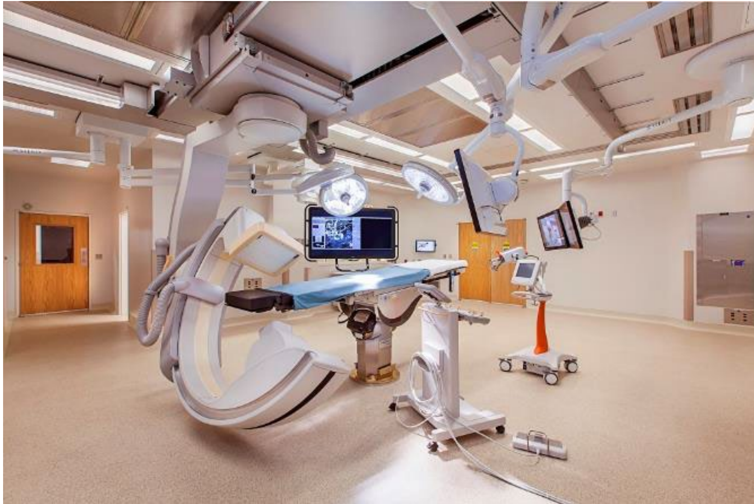
VAMC DETROIT OPERATING ROOM, MONOPLANE HYBRID 900 NSF
