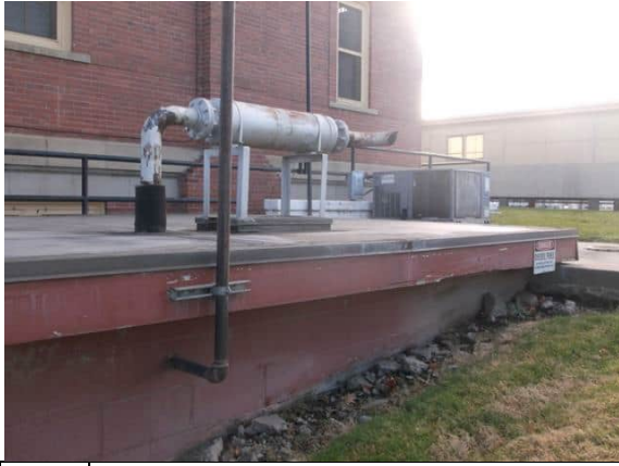
Photo #21: Looking south at the emergency generator and diesel UST location north of Building 78
