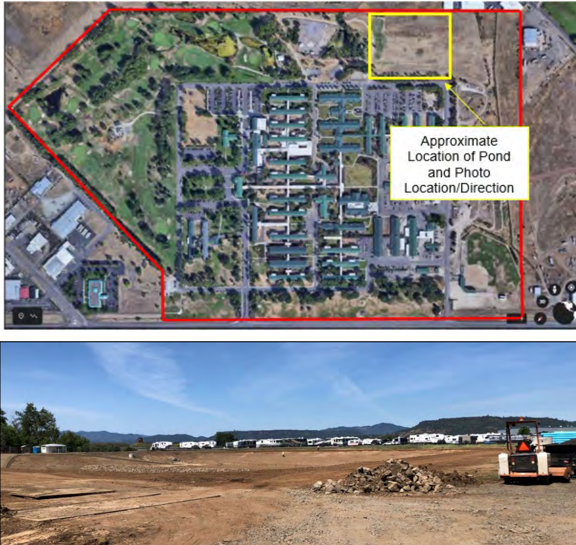
Figure 3-3 Approximate Location of the Stormwater Retention Pond (prior to construction) and Photo of Pond (May 11, 2021)
