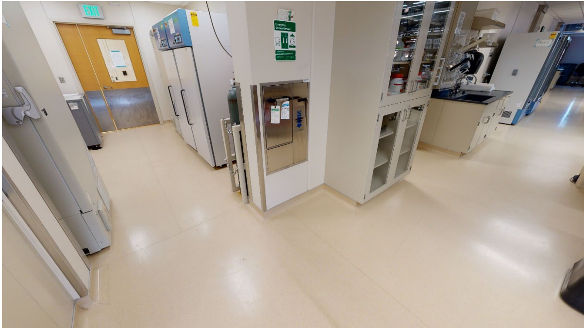
Image A.5 The Emergency Shower / Eyewash Station is centrally located in the biomedical laboratory at the Rocky Mountain VAMC R&D Facility.
