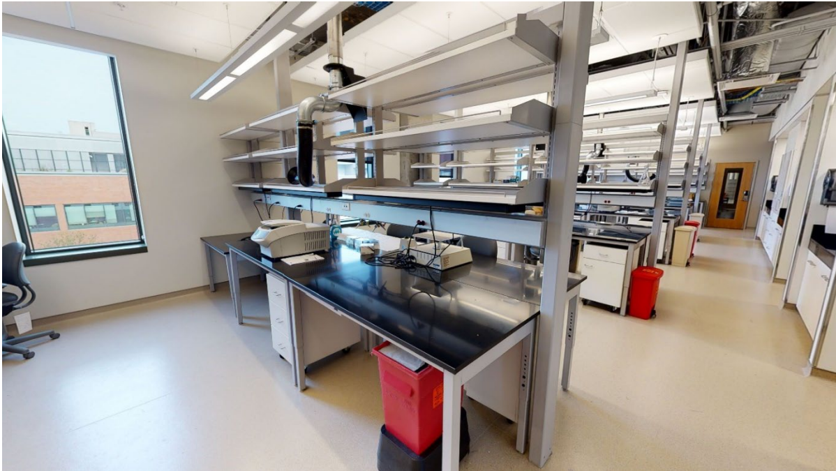
Image A.14 The adaptability of the Lab Bench Units at the New Orleans VAMC R&D Facility is enhanced with snorkel exhaust systems.
